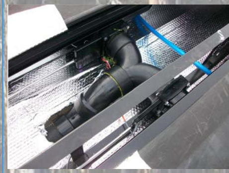
Heated Holding Tanks With Protected Valve System
